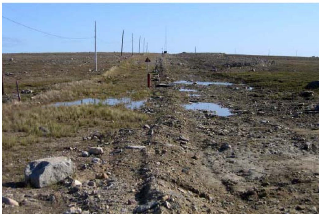
Figure 14. Surface water ponding adjacent to the buried water pipeline near the water supply lake. Surface water leads to saturation of underlying sediments and the seasonal formation of ice layers, resulting in increased ground heave.
