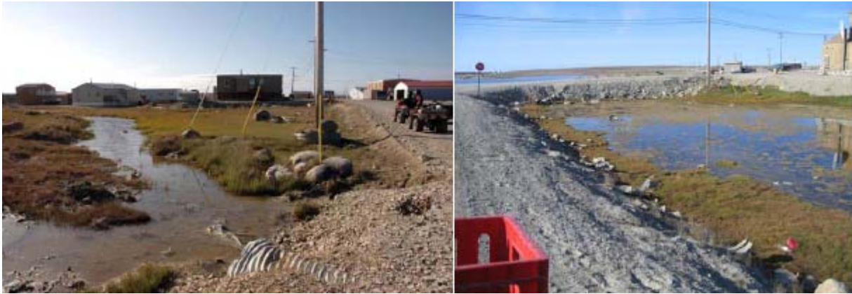
Figure 13. Examples of ponded surface water in Cambridge Bay owing to improper grading or positioning of drainage culverts.
